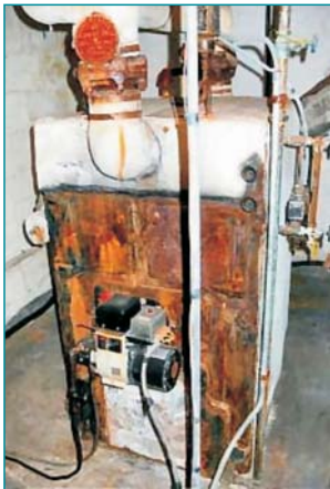
Old Boiler in Need of Replacement
