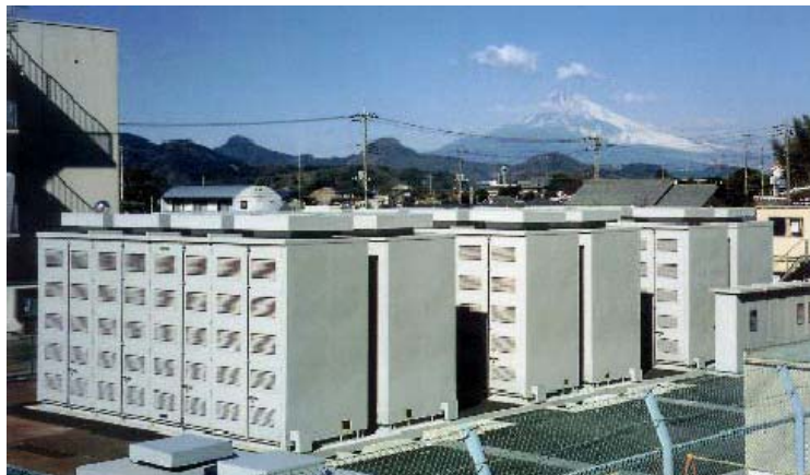
Figure 3.7 6MW, 8h NaS battery storage system
