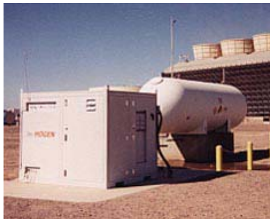
Figure 3.813 PEM electrolyser and storage vessel
