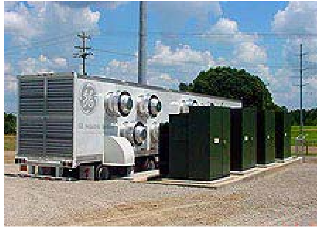
Figure 3.5 Distributed SMES at a substation
